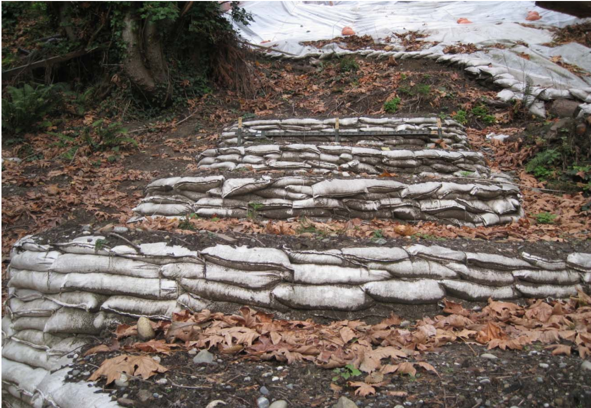
Photo #7: View of the upper tiered sandbag walls on the project site (Nov 11 2016).
