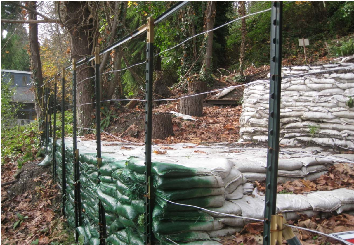
Photo #2: View of one of the sandbag retaining walls on the lower part of the slope (Nov 7 2016).
