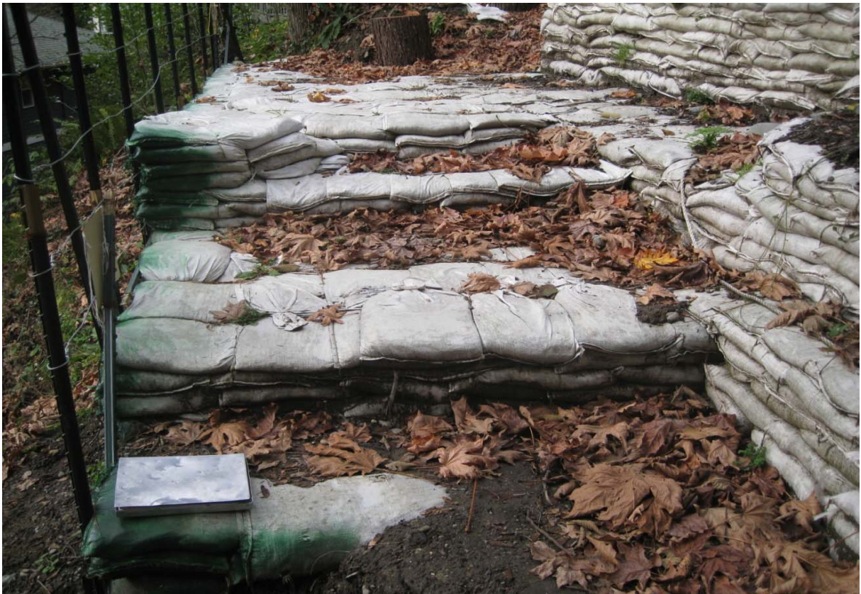
Photo #4: View of one of the sandbag retaining walls on the lower part of the slope (Nov 11 2016).
