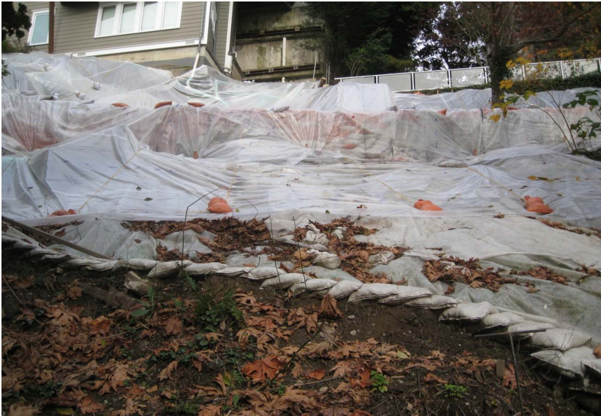
Photo #13: Sandbag berm and plastic sheeting on northern margin of site and adjacent properties (Nov 11 2016).
