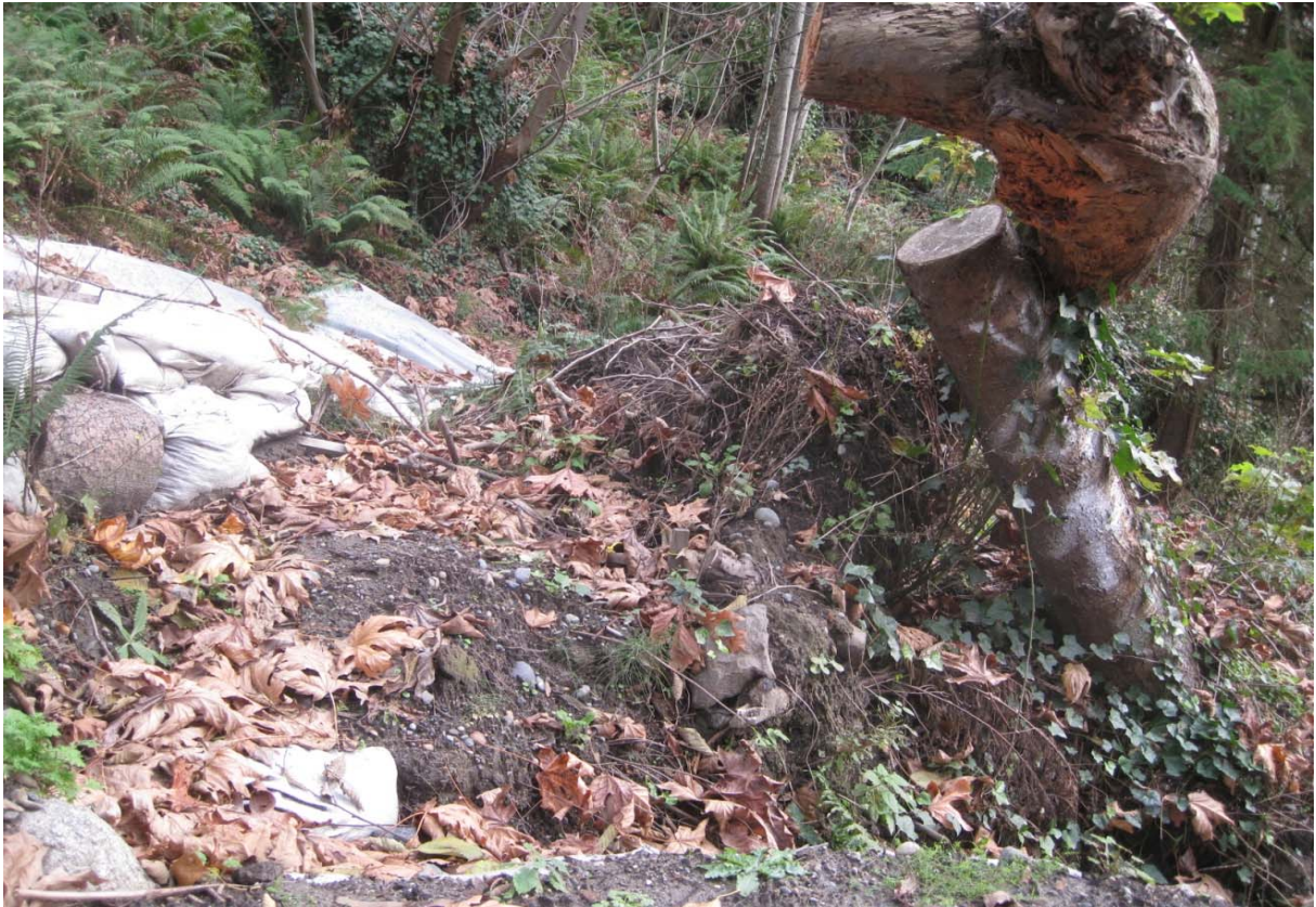
Photo #9: Eastward view across slope above tiered sandbag walls, north margin of project site (Nov 11 2016).
